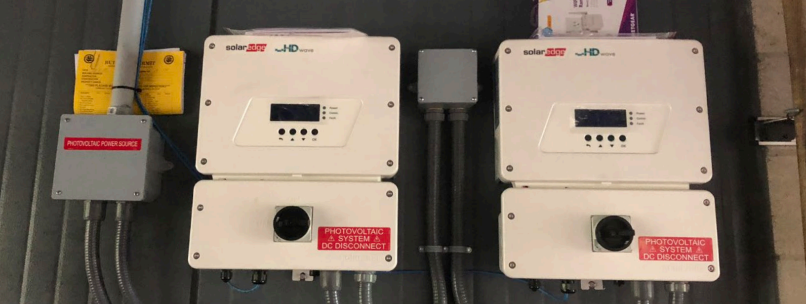
Two inverters that convert the DC electricity produced by the solar system into AC to power the home.
