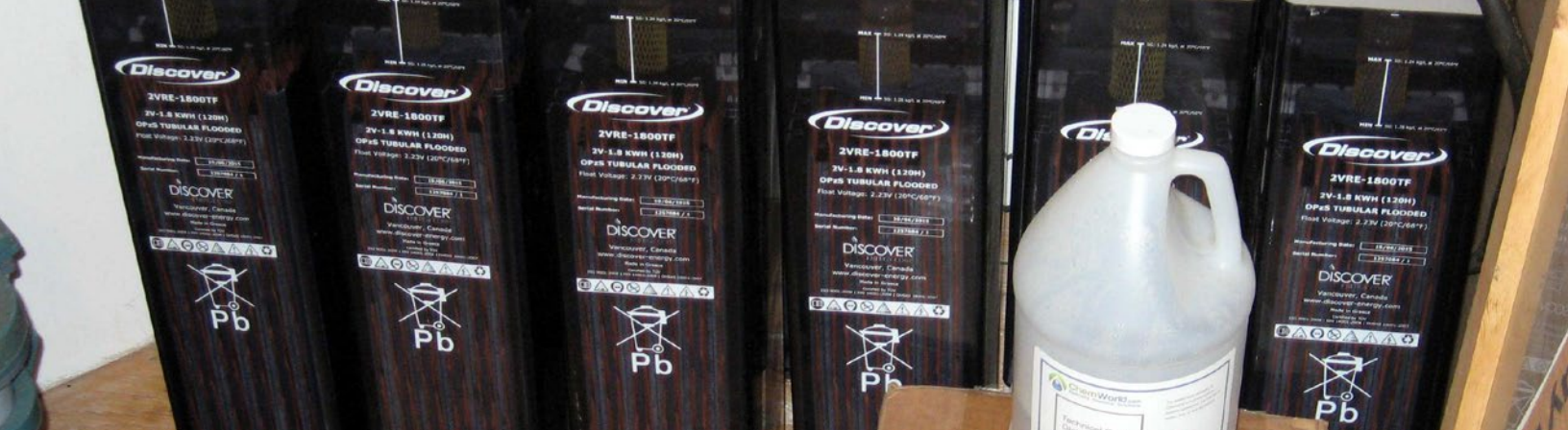
Example of a lead acid battery bank.
