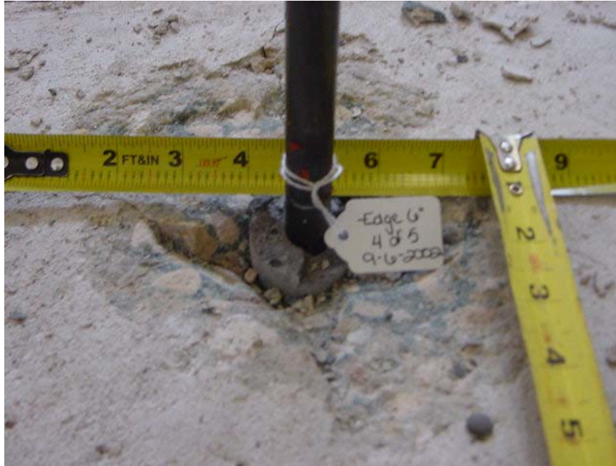
Figure E-7 Typical grout/concrete bond failure of single core-drilled anchor installed 6.0 inches from one edge with grout plug
