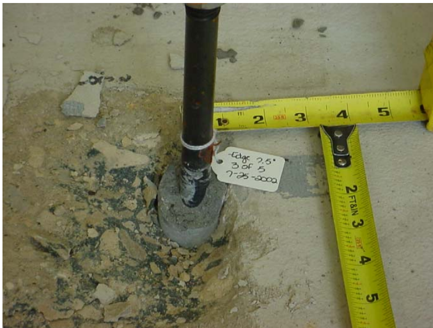
Figure E-8 Typical grout/concrete bond failure of single core-drilled anchor installed 7.5 inches from one edge with grout plug
