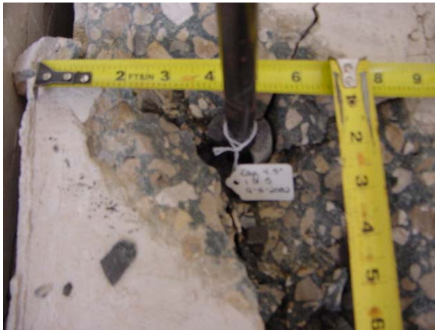
Figure E-6 Typical grout/concrete bond failure of single core-drilled anchor installed 4.5 inches from one edge with grout plug and diagonal cracking of surrounding concrete
