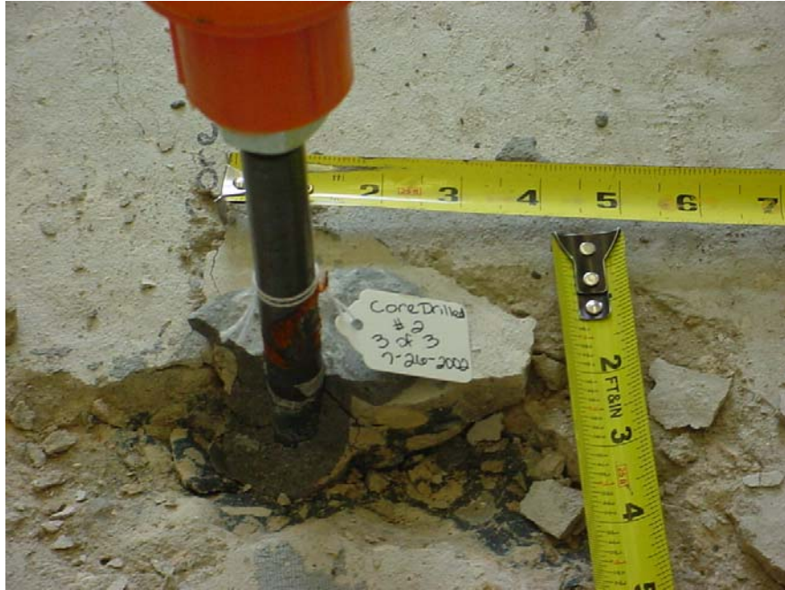
Figure E-3 Grout/concrete bond failure of single core-drilled anchor with secondary shallow cone removed and grout plug exposed
