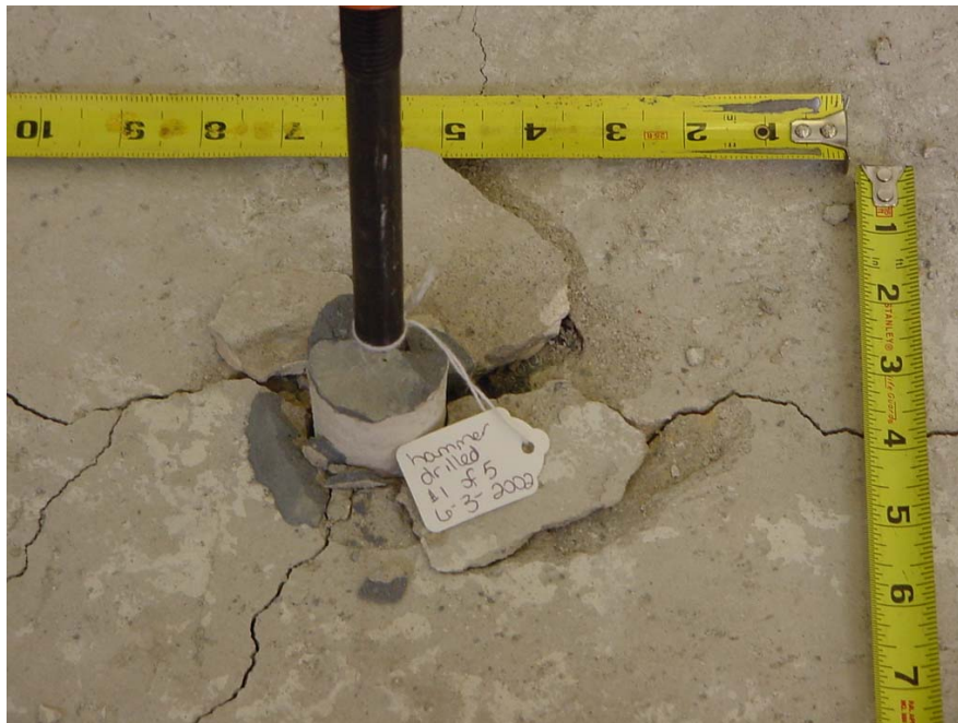
Figure E-4 Typical grout/concrete bond failure of single hammer-drilled anchor with grout plug
