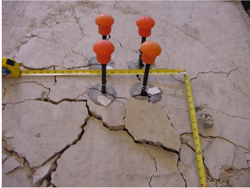
Figure E-9 Typical surface view of cone failure of quadruple fastener anchor group with anchor spacing of 5 inches
