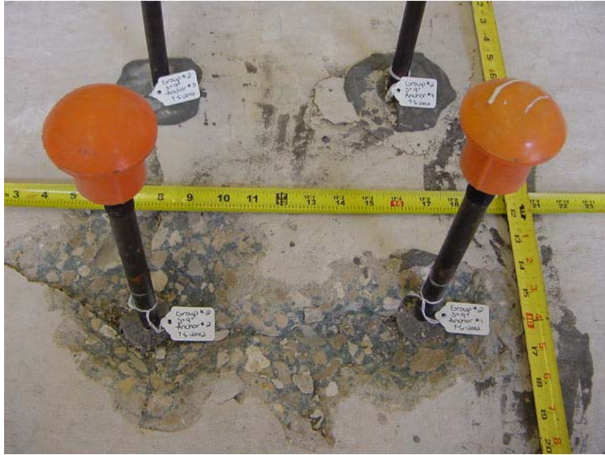
Figure E-11 Typical grout/concrete failure of quadruple fastener anchor group with anchor spacing of 9 inches
