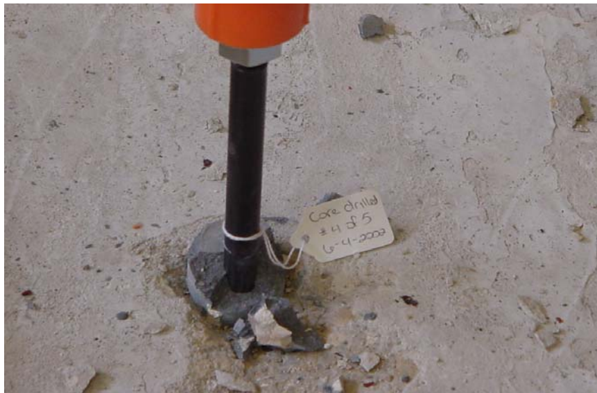
Figure E-1 Typical grout/concrete bond failure of single core-drilled anchor with grout plug
