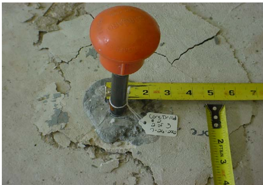
Figure E-2 Typical grout/concrete bond failure of single anchor with secondary shallow concrete cone
