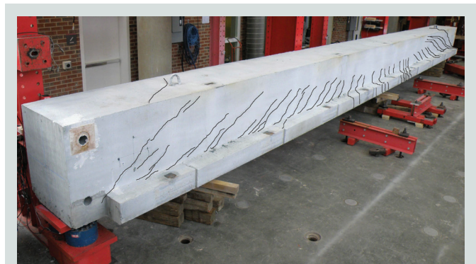
Figure 5. Inner face cracking observed after failure for a control compact L-shaped beam with closed web reinforcement (LG1). Note: Cracks are digitally enhanced.
