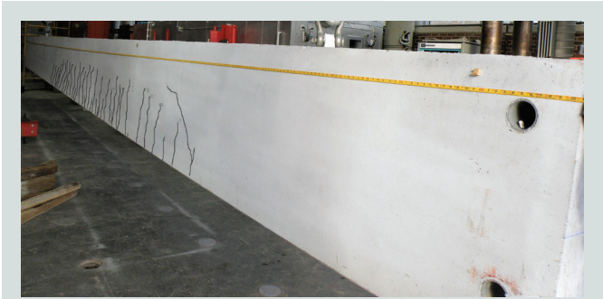
Figure 8. Typical outer face cracking in a compact L-shaped beam (LG1). Note: Cracks are digitally enhanced.
