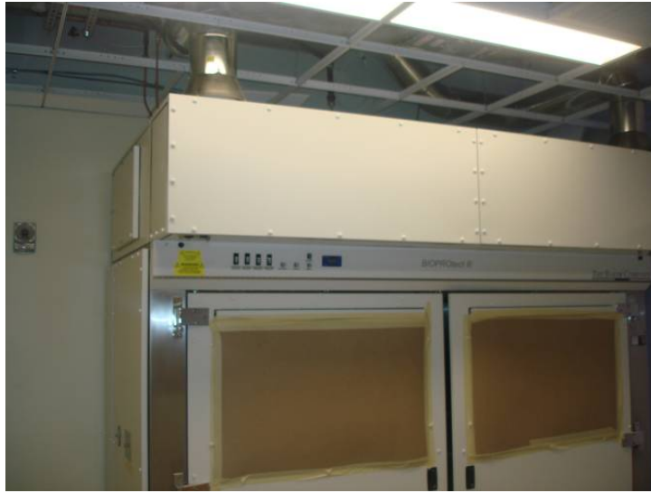
Figure 26: Pre-piped gas line with Fume hood assembly
