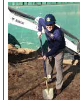
Brian Raney, BS 05, at the groundbreaking of UC Berkeley's Hellman Tennis Complex upgrade project in January.
