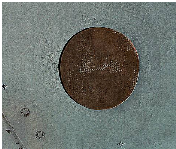
Figure 13. Composite-Bonded Patch Failure Showing Interfacial Failure Between Adhesive and Patch Surface due to Presence of a Silicone Release Agent on Peel Ply 2
