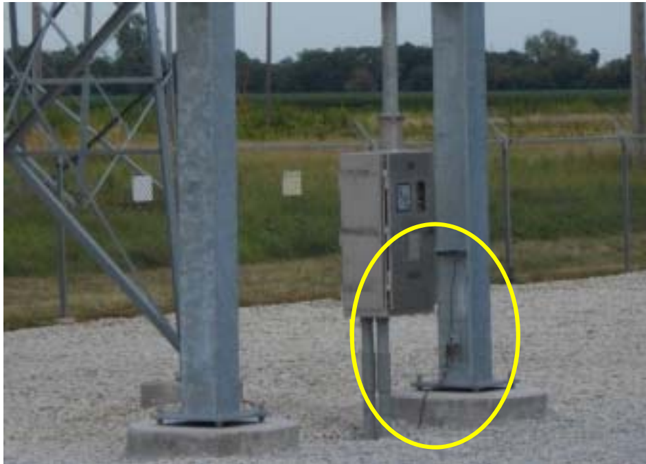
Figure B2 - Above-grade Grounding on Steel Structure (Watts Electric 2015)
