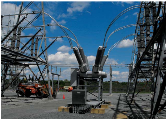
Figure B6 - High-voltage Circuit Breaker; Gas Type (Utility Products 2014)
