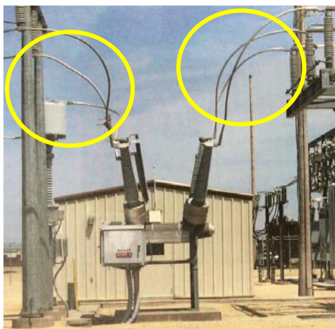
Figure B5 - Jumpers to Circuit Breaker (University of Wisconsin-Madison)
