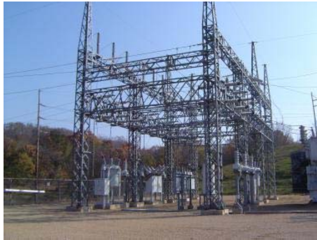
Figure B12 - Steel Lattice Structure for Ring Bus Configuration (Heinemann et al. 2012)
