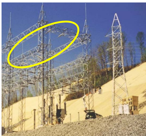
Figure B4 - Lattice Box Structure with Strain Bus (Fabriment 2008)
