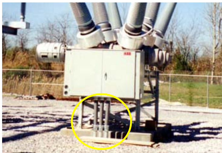
Figure B1 - Above-grade Conduit to Breaker Cabinet (Commonwealth 2015)
