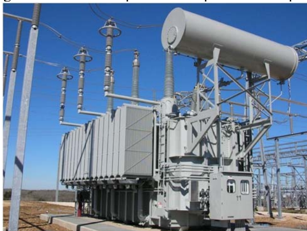
Figure B8 - Example of a High-voltage Power Transformer (Newhart Services 2015)
