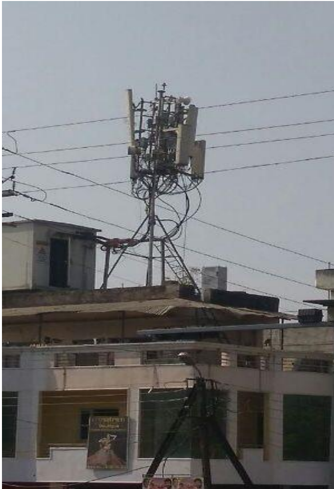
Conventional Telecom Tower
