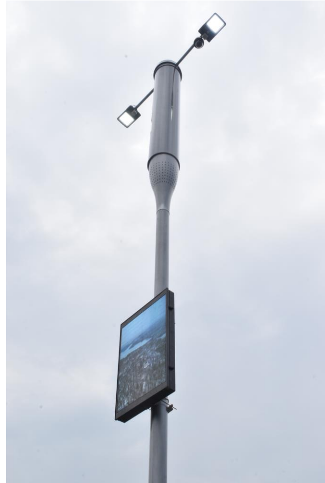
Installed Smart Pole
