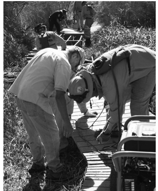
Jerry Messerschmidt directs a CalFire crew in repairing the Mesquite Trail boardwalk
