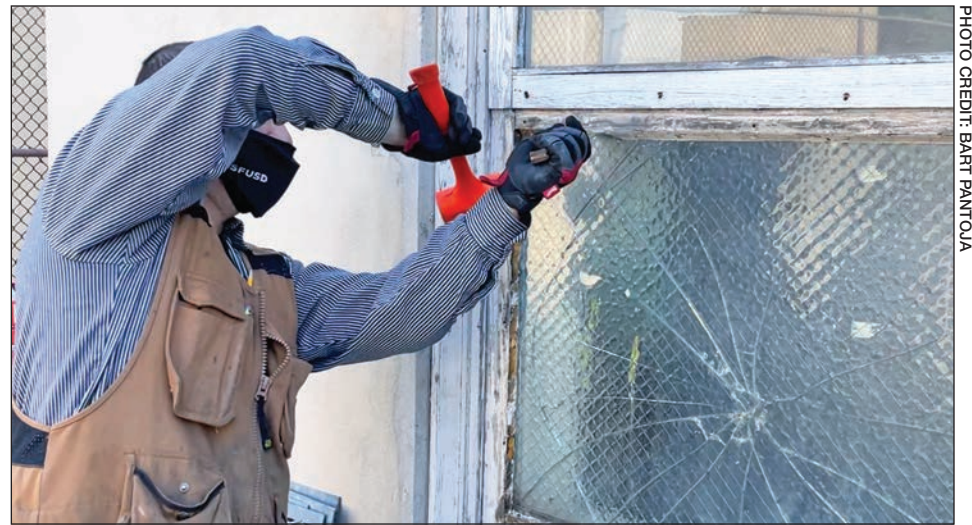
Armando Hernandez, journeyman glazier with Glaziers Local 718, takes the first step to remove a window at Mission High School in June 2021.
