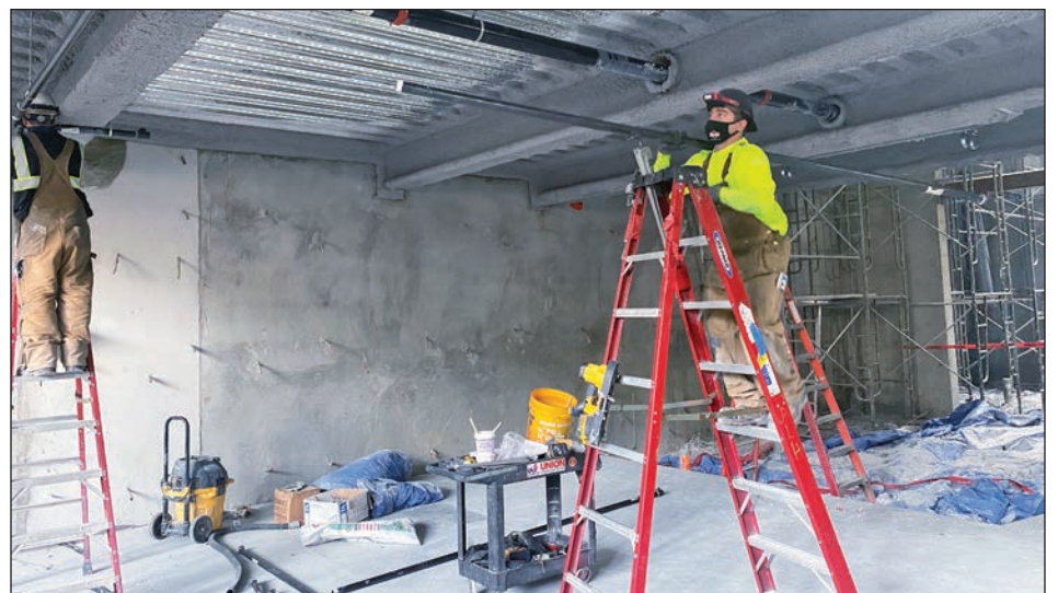
Foreman Vince Copeletti, a sprinkler fitter, installs piping for a sprinkler system.
