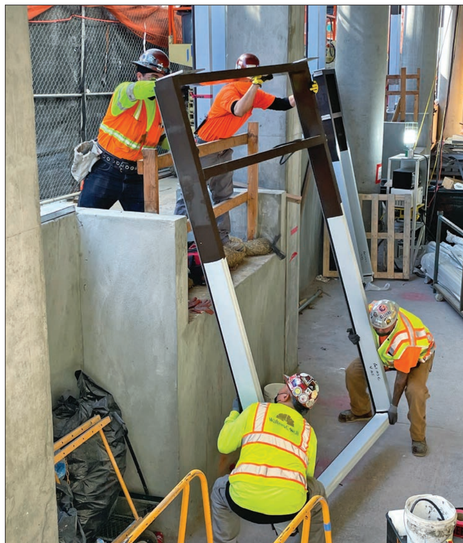
On the Job: Highrise Glass is wrapping up the project at 1001 Van Ness. Check brothers from LU718, LU169, and LU1621 on site. Brothers Johnny, Manny, Kevin, and Jose are installing some frames in the lower lobby on the Van Ness side of the building.
