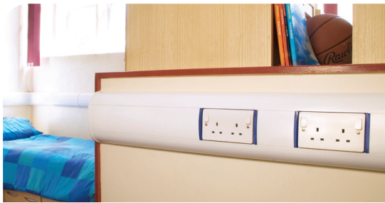
Odyssey trunking with Part M boxes installed at Old Swinford Hospital School, Stourbridge.
