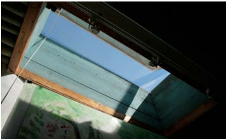
Open skylight without wire covering
