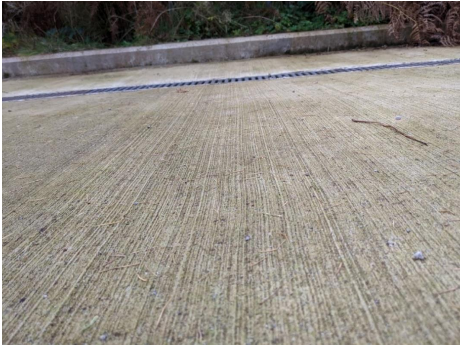
Image: Example of concrete with rake markings sloping towards the drainage point.
