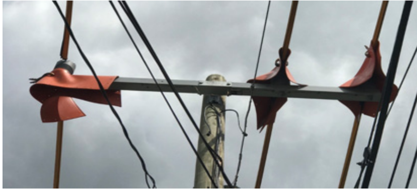
Lindsey sensors being installed on energized distribution feeder
