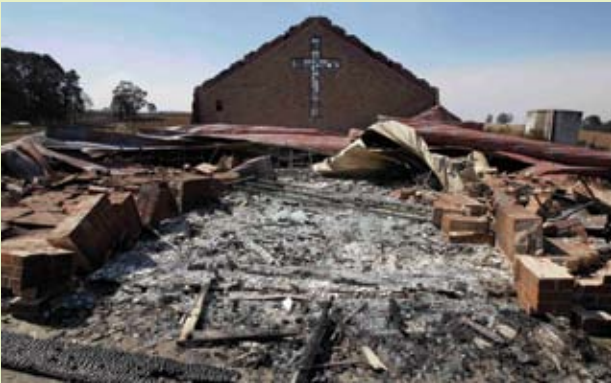
BEFORE: St Mary's Church, Kinglake was completely destroyed in the Black Saturday bushfires, parishioners came across the remains of the tabernacle in the burnt rubble.
