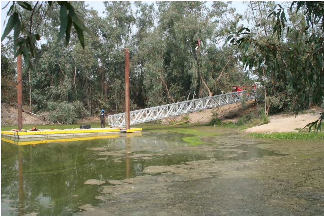
Figure 3: Fishing Pier during installation of the walkway. Also notice the low water level from before the installation of the French Drain structure.
