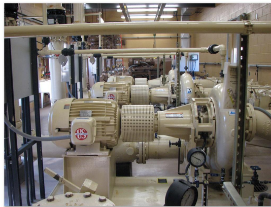
Existing RAS/WAS Pump Station
