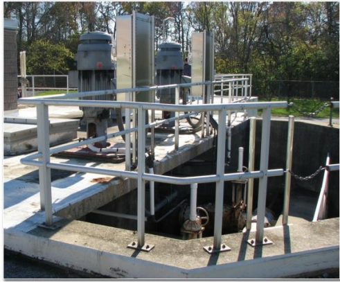
The (2) Existing Vertical Turbine Pumps
