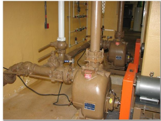
The (2) Existing Grit Pumps
