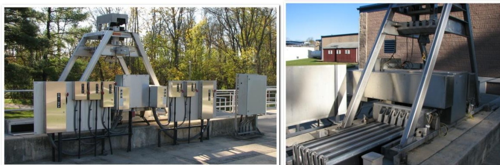
Existing Ultraviolet Disinfection Unit
