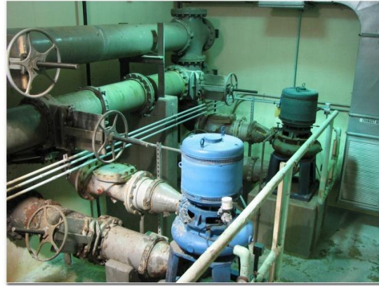
(2 of the 5) Existing Dry Pit Pumps
