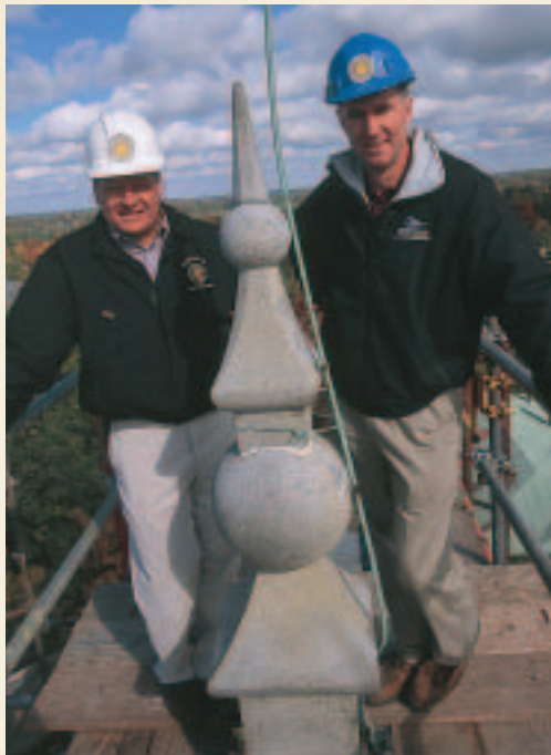
Chapel restoration project manager Don Borkowski of the Bowdoin facilities department (right) and fellow facilities project manager Jeff Tuttle (left) have an inspiring view from the tip-top of the Chapel’s north tower. Some 150 years after the Chapel was constructed, Bowdoin has returned to the original Brunswick quarry for the granite needed to repair the time-worn towers..
