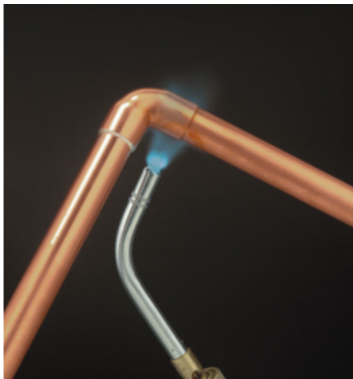
Brazing, shown above, generally involves air settling swirl or oxyfuel torches due to higher temperatures used to melt filler metals.
