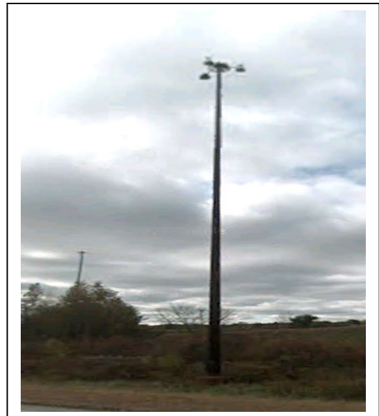
Typical NHDOT High-mast Light Poles
