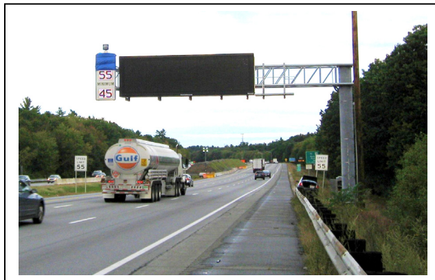
Typical NHDOT DMS Overhead Structure
