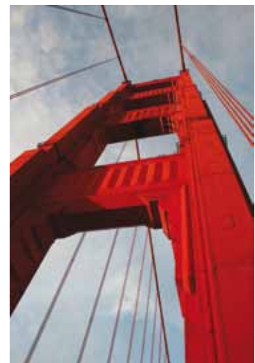
Figure 6 The south tower of the Golden Gate bridge constructed from steel. ( http://en.wikipedia.org/wiki/File:Golden_Gate_bridge_pillar.jpg )
