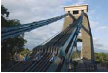
Figure 7 The cables of the Clifton Suspension Bridge are made from wrought iron. The Bridge was designed by Isambard Kingdom Brunel and was opened in 1864. ( http://upload.wikimedia.org/wikipedia/commons/3/3a/Uk_bristol_csbchains.jpg )
