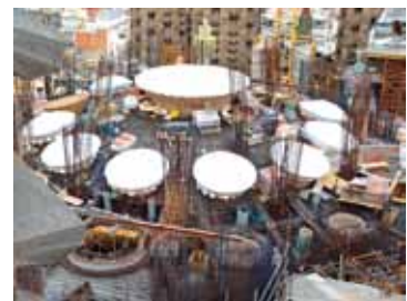
Figure 9 – Complex network of rebar in the roof of the Sagrada Familia in Barcelona prior to concrete pouring. ( http://en.wikipedia.org/wiki/File:SagradaFamiliaRoof2.jpg )
