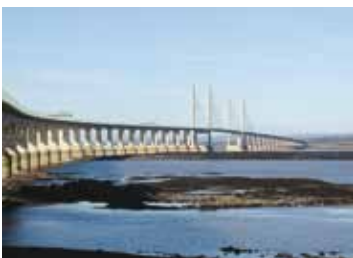
Figure 2 Second Severn Crossing comprises two approach bridges separated by a cable-stayed section over the shipping channel. ( http://en.wikipedia.org/wiki/File:New_severn_bridge_best_750pix.jpg )
