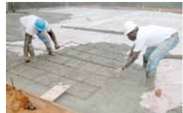
Figure 8 – Installing a steel mesh in to a wet concrete floor raft to provide reinforcement. ( http://upload.wikimedia.org/wikipedia/commons/0/04/Concrete_rebar_0030.jpg )
