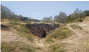
Figure 1 Bronze Age Arkadiko Bridge in Greece. Built by the Myceneans on the road from Tiryns to Epidaurus it dates from 1300 BC and is still used today. ( http://www.panoramio.com/photo/13255844 )
