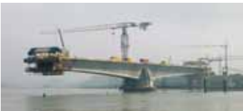
Figure 3 Construction of the Pierre Pflimlin Bridge on the border between Germany and France began in the late 1990s and the crossing was opened in 2002.. ( http://en.wikipedia.org/wiki/File:Pierre_Pflimlin_Bridge_UC_Adjusted.jpg )
