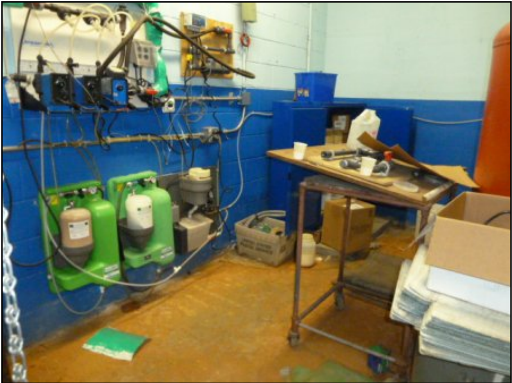
Chiller treatment chemicals
