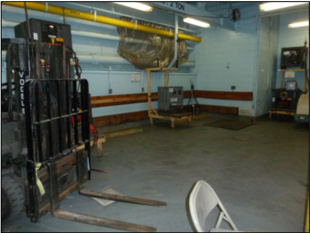
Battery recharge room
