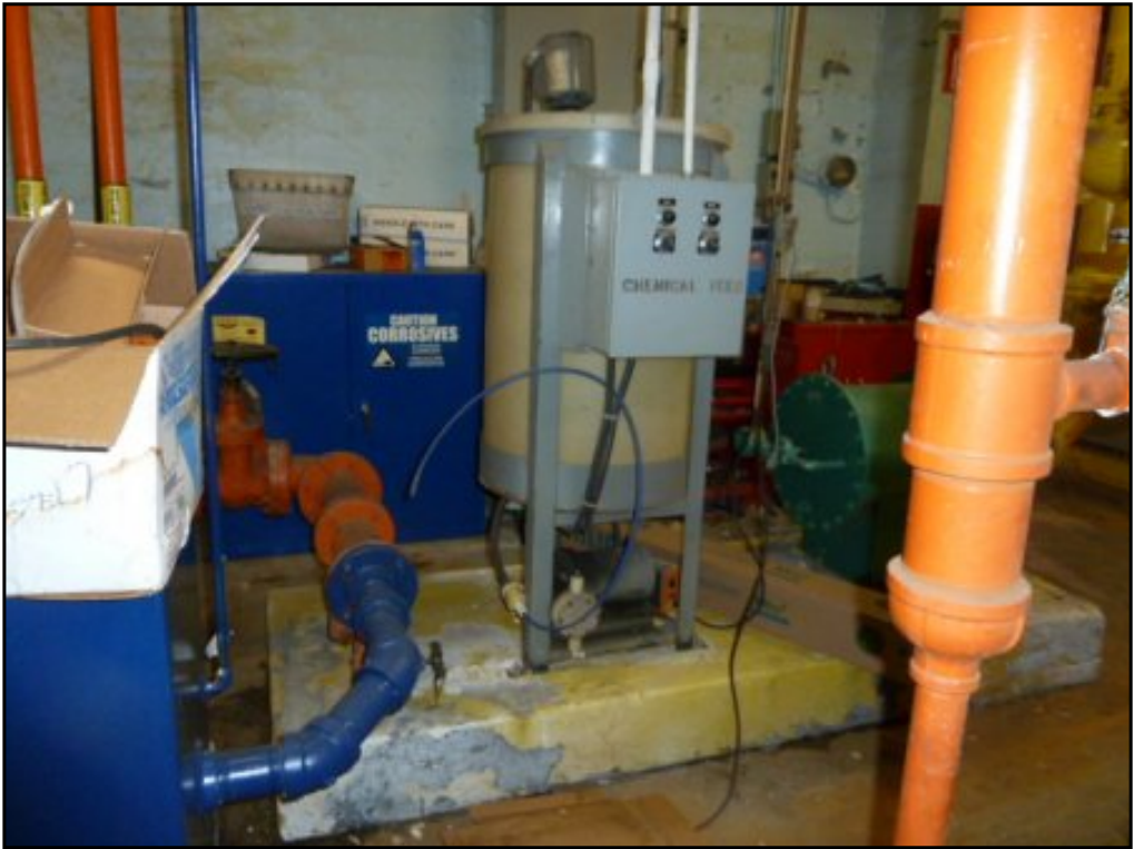
Boiler feed chemicals
