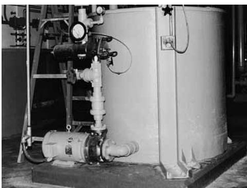
Reverse osmosis, Ósmosis invertida
