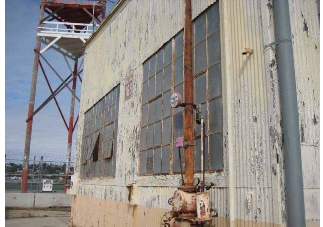
Building 166 - Salvage Headquarters, detail of window on West Elevation, San Diego, California, October 2009.
