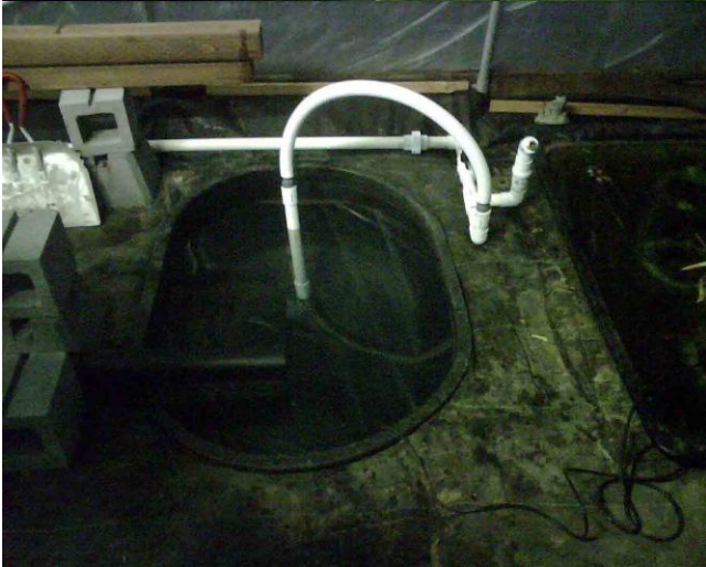
Bell Siphon drain tube - - which flows down and - - empties into the sump tank
