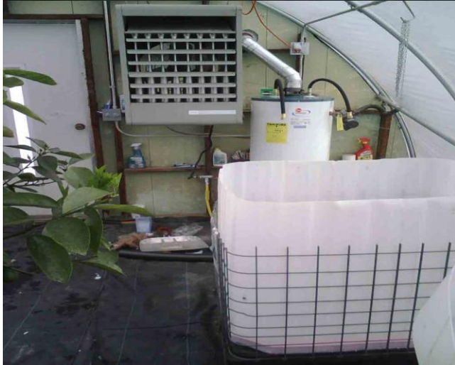
275 Gallon IBC Tote, top cut off for the fish tank - - - Propane Water Heater to heat water
