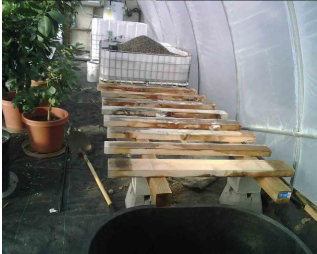
Beds filled (leveled first) - - - - - Base for Floating Raft System- dump tank below
