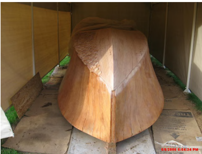
“Mahogany sheathing strips are being installed on the bottom of the hull.”
