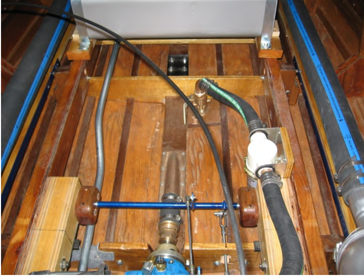
“Raw water pickup and filter.”
