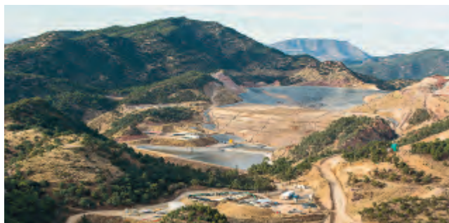
AT LA INDIA , construction of the new leach pad was completed within budget and preparation activities for the start-up of mining at the Main Zone pit were also completed in 2015.
