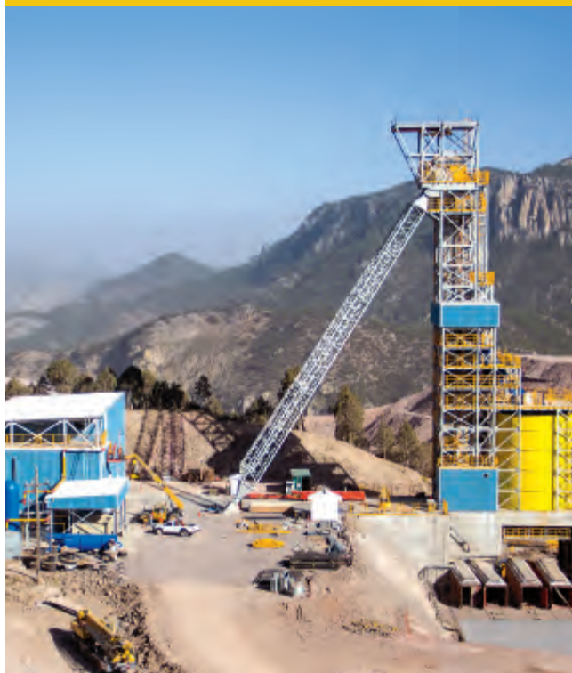
COMMISSIONING OF THE PINOS ALTOS SHAFT in 2016 will allow better matching of the future mining capacity with the mill once the open pit mining operation begins to wind down.
