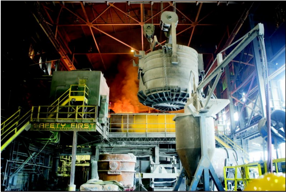
Using hardware and software from NI, Nucor developed a variety of automation systems that have greatly reduced the amount of electricity used and eliminated potential safety issues at its Marion, Ohio facility.
