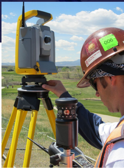
Surveyors used the Trimble S6 Total Station to complete the closed loop traverse of the new building site.
