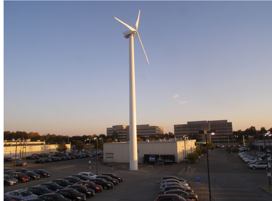
Northwind 100kW; Byers Group Mazda/Subaru Dealership in Columbus OH. Photo from Byers and Renier Construction, NREL/PIX 18221
