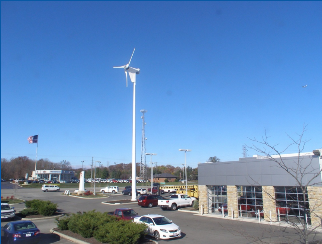
15kW Proven; Byers Group Toyota Dealership in Delaware OH. Photo from Byers and Renier Construction, NREL/PIX 18222
