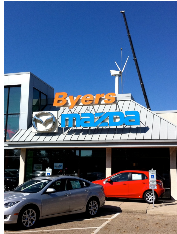
Installation of 100kW, 15KW Northwind Turbine at Byers Automotive Group in Columbus OH, Renier Construction builder. Photo from Byers and Renier Construction, NREL/PIX 18821
