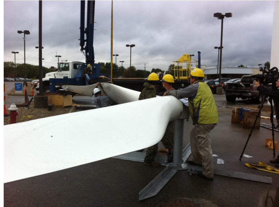
Installation of 100kW, 15KW Northwind Turbine at Byers Automotive Group in Columbus OH, Renier Construction builder. Photo from Byers and Renier Construction, NREL/PIX 18815
