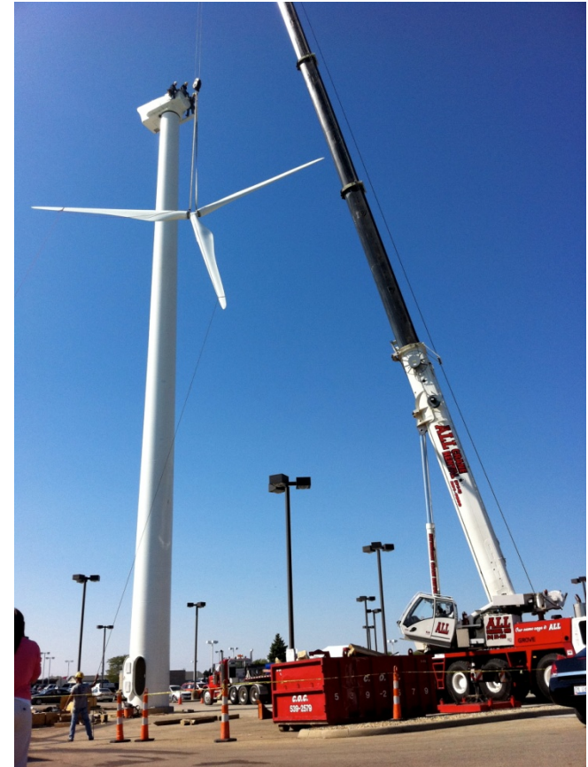
Installation of 100kW, 15kW Northwind Turbine at Byers Automotive Group in Columbus OH, Renier Construction builder. Photo from Byers and Renier Construction, NREL/PIX 18820
