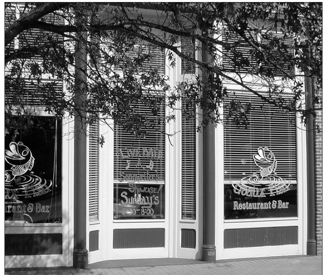
Maintain recessed entries where they are found. This recessed form, for example, preserves the original character, even though it no longer serves as a doorway.
