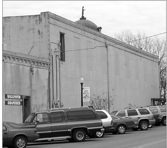
The upper-story windows on the side of this historic commercial building have been filled in with brick. Where instances like this exist, consider reopening the windows.
