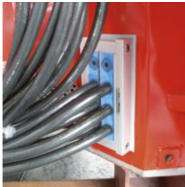
Light railway vehicle: The fire rated Roxtec CF 24 F1 helps ensure passenger safety by preventing the spread of fire into the passenger compartment.
