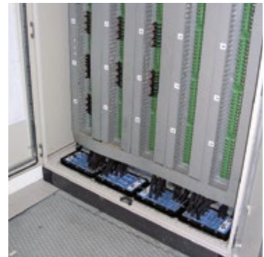
DCS/PLC and I/O marshalling cabinets: Roxtec solutions reduce required cabinet space, ensure functionality and provide capacity for additional cables.
