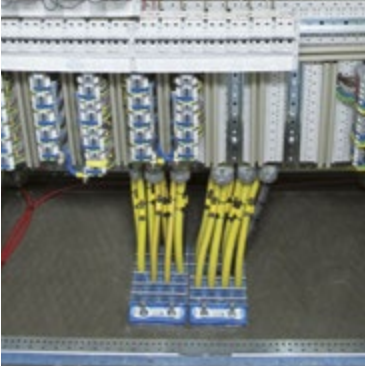
Transformers and switchgear: The Roxtec GHM solution provides protection to ensure operational reliability.
