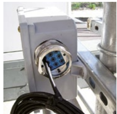
Telecom cabinet: The Roxtec RG M63 cable glands are weather, water, pest and dust tight.
