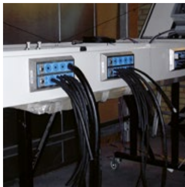
Wind turbine: Roxtec transits for potential equalization as well as the Roxtec standard system for control cabinets in the nacelle.
