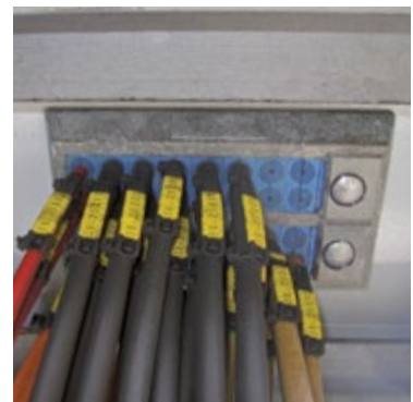
Instrumentation and communication: The Roxtec CF 32 provides protection against coal dust.
