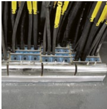
Radio room: RFI shielded EMC and firestop solutions for radar and navigation equipment in bulkheads.
