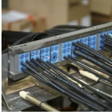
Driver cab and engine room: Customized sealing solution installed to keep tight between the driver cab and engine room.
