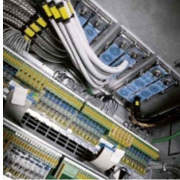
I/C cabinets: Neat and area efficient cable entry seals suitable for safety and non-safety applications.
