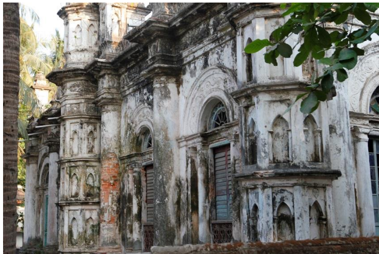
☹️ ↑ Sittwe's once imposing main mosque has fallen into a state of disrepair and decay. Shuttered since 2012, police guards and barbed wire fences prevent anyone from entering, March 2016. ©Amnesty International.
