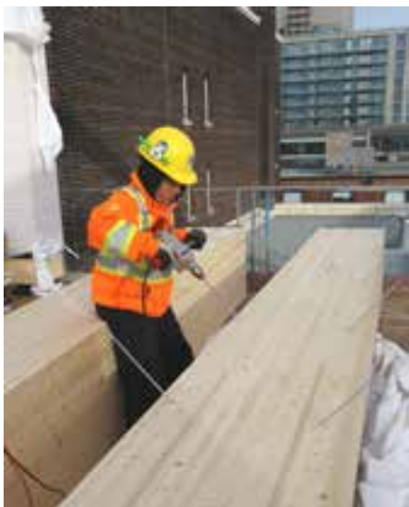
Carpenter uses 600mm screws to stitch together two pieces of glulam to complete the assembly of a beam prior to its installation.
