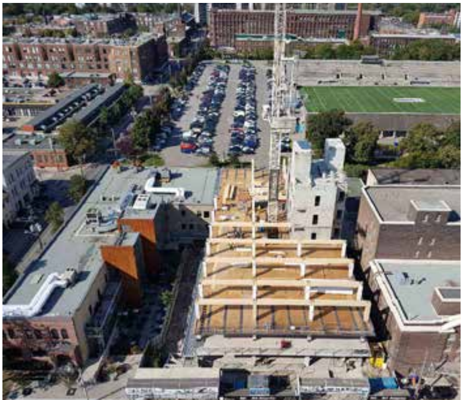
Bird's-eye view of 80 Atlantic during the installation of the timber columns and beams for the third floor.
