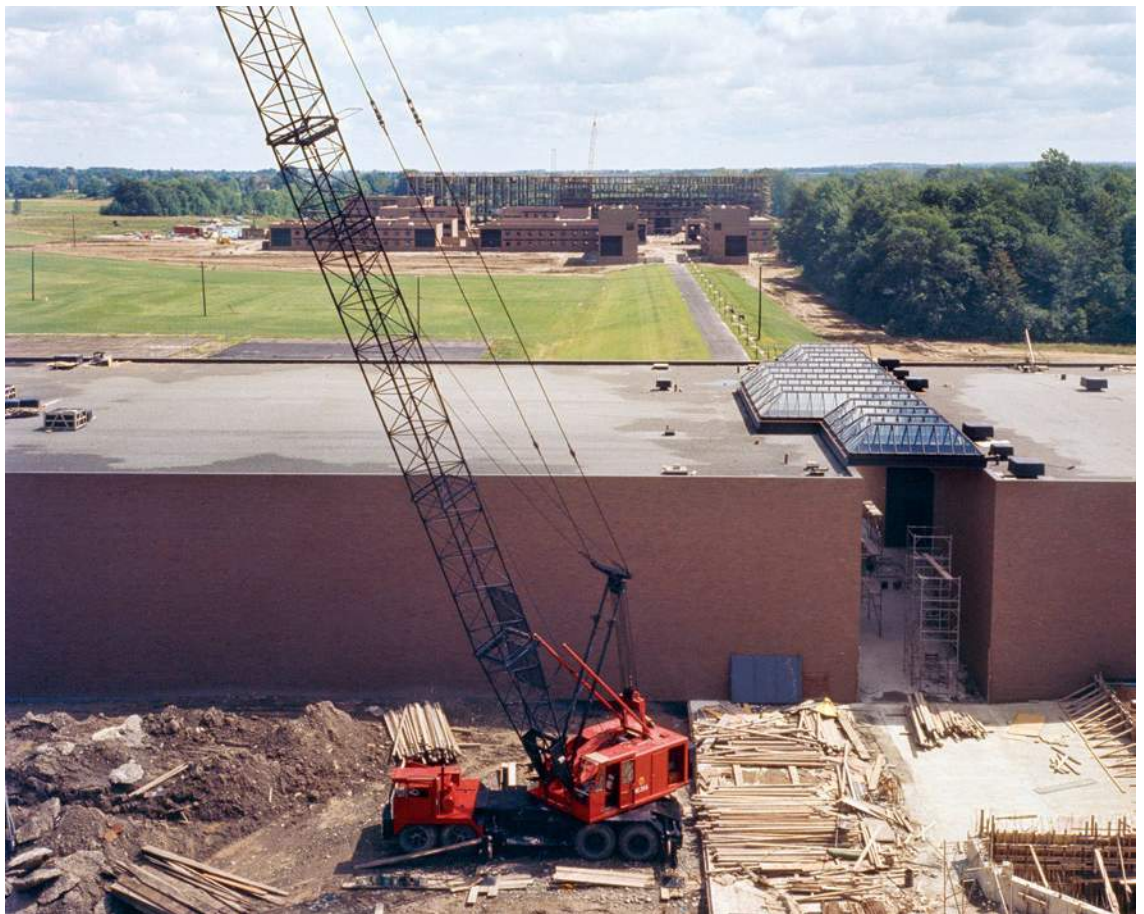
Planning and construction of the Henrietta campus lasted seven years. From top left clockwise, varying stages of construction can be seen on the Frank Ritter Memorial Ice Arena, Clark Gymnasium and what is now Thomas Gosnell Hall, which houses the College of Science.
