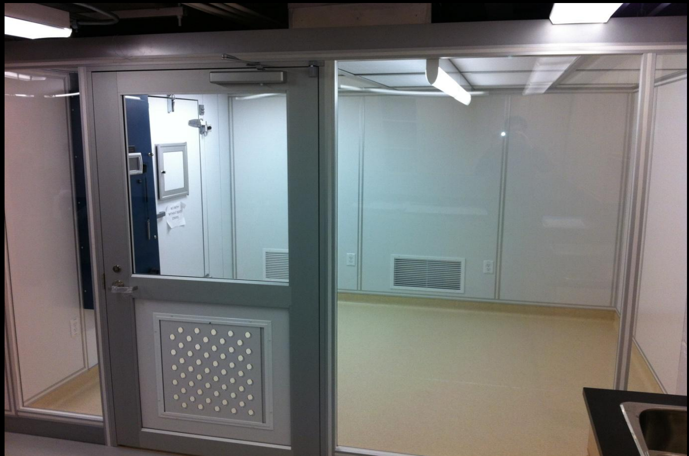
Class 1000 clean anteroom, with door to environmental chamber (at left); University of Alberta
