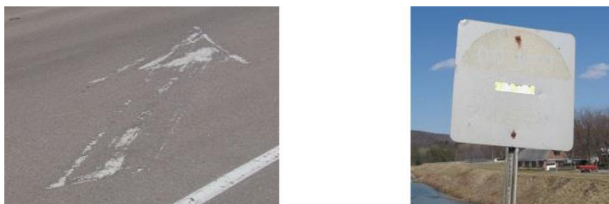
Figure 5.6.16–1: Examples of Poorly Maintained Pavement Marking and Signage
