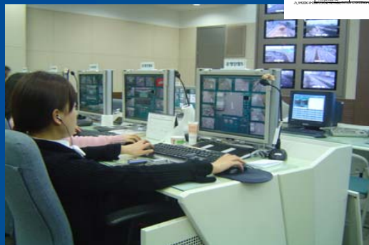
Remote Control Centre
