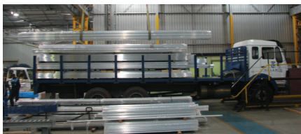
Use correct crane and slings for lifting, hoisting and loading
