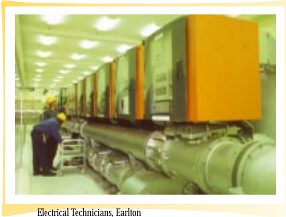
Electrical Technicians, Earlton Bramble and Kurt Hislop, test the relay systems on switchgear equipment in the new 69KV gas-insulated switchgear substation which was completed in summer 2000.
