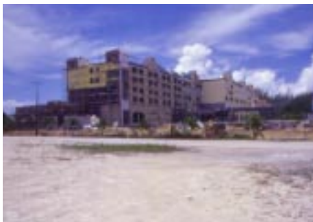
Construction is well underway on the 232-room Holiday Inn Resort overlooking Seven Mile Beach which is due to open in November 2000. The hotel's bar and dive shop is located on the beach.
