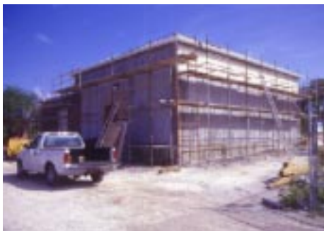
The new 69KV South Sound substation is due to be completed later this year as part of our transmission and distribution expansion programme.
