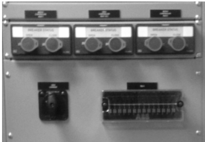
Fig. 9. Control switch module with indication located in the control house.
