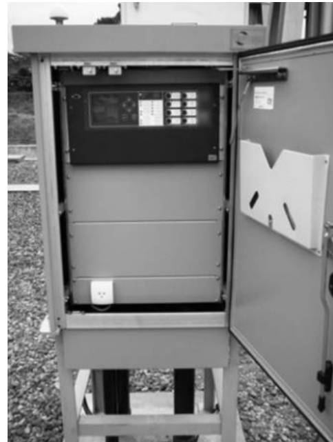
Fig. 10. Typical IED field kiosk installation.
