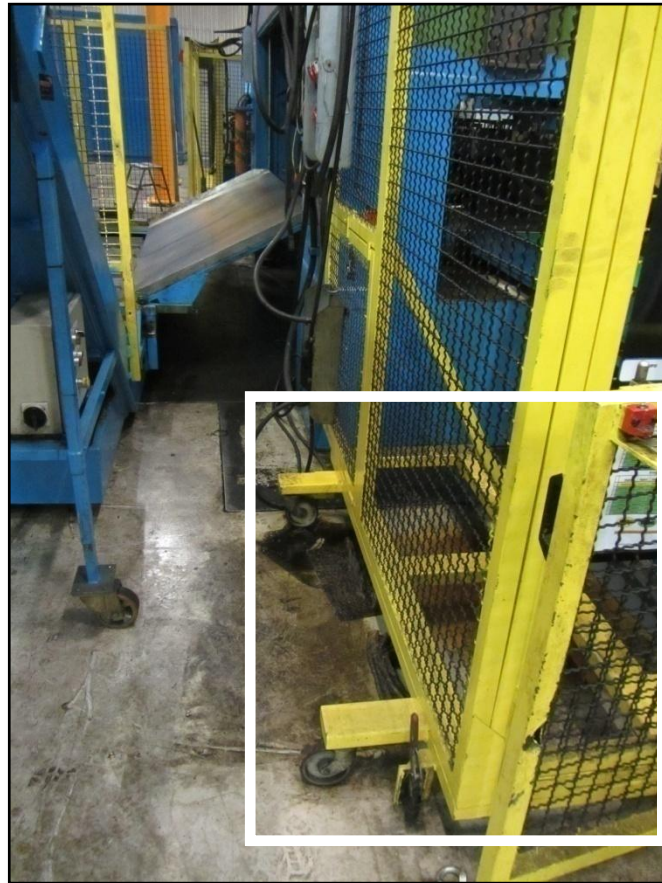
Figure 38: Protection fence legs
