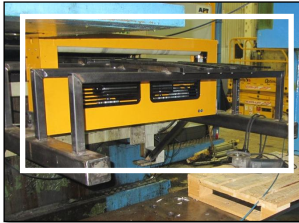
Figure 32: New feeder installation
