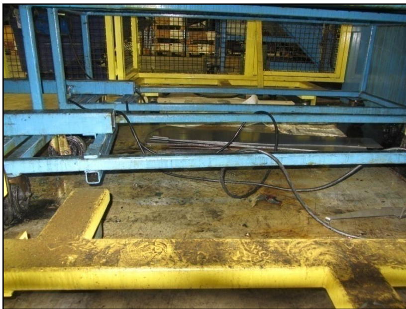
Figure 37: View under the conveyors
