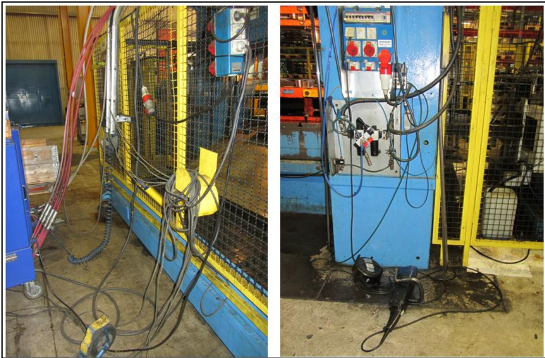
Figure 42: Wires and messy area
