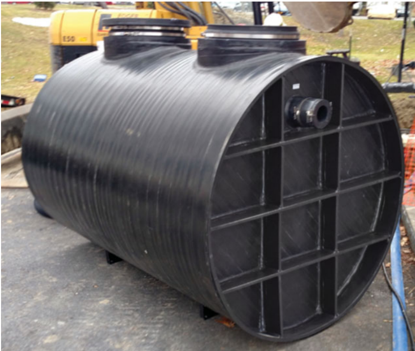
GGI-1000 prior to installation at a university cafeteria
