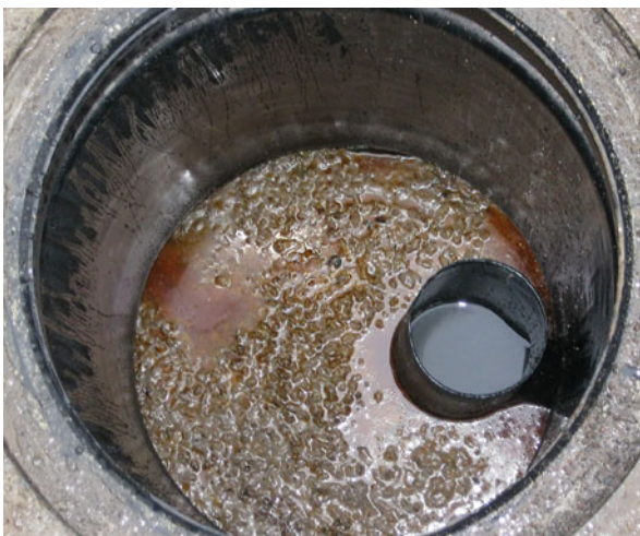
top view of GB-250 outlet diffuser in service
