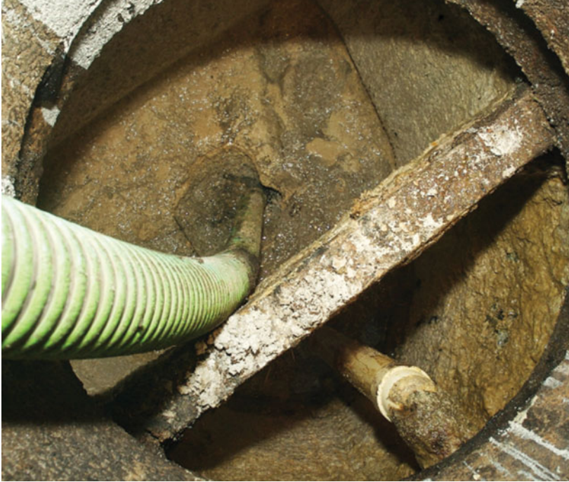
concrete units corrode and require replacement every 10 years (avg.)
