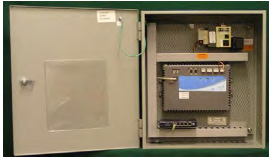
PAGx0000xAC0 NAE Standard Control Panel Assembly Mounted in a 20 in. x 24 in. Enclosure
