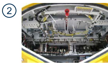
Replacement Avionics Shelves
