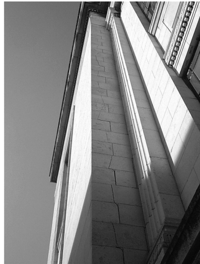
Figure 4: Cracking of cladding due to corrosion.
