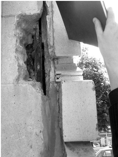
Figure 3: Corrosion of steel frame.
