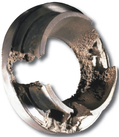
Conventional valve trim destroyed by high velocity-induced cavitation
