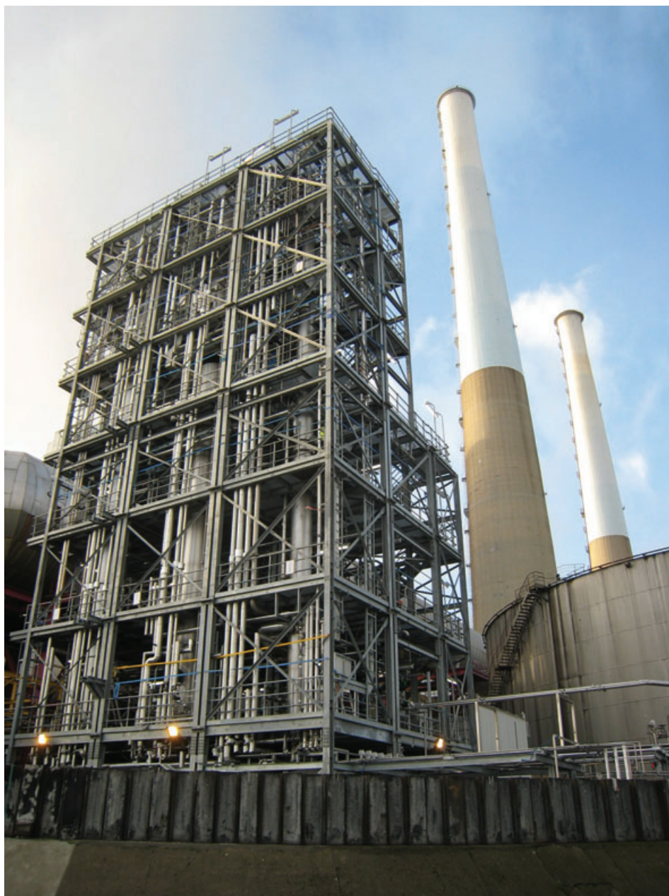
Figure 2 - the EdF Le Havre demonstration unit features the latest Advanced Amine Process design for the absorber, regenerator and thermal management systems and will reduce energy consumption and minimize solvent degradation.
