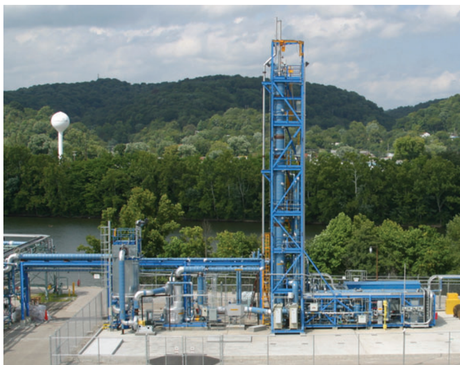
Figure 1 - The AAP pilot plant facility in Charleston, West Virginia, U.S. is capable of capturing 5 tonnes of CO 2 per day
