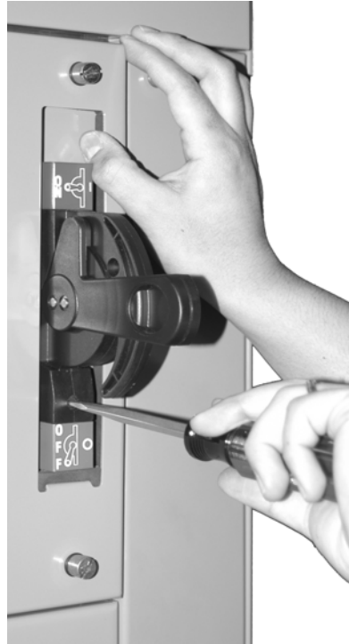
Figure 27 - Operating Handle Defeater for Vertical Operator Handle
