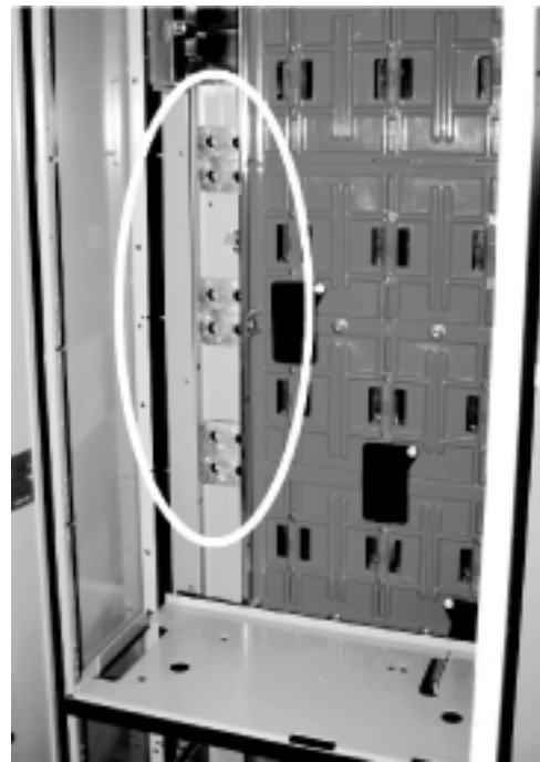
Bus Splice Access Cover Removed
