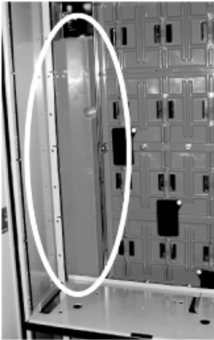
Bus Splice Access Cover In Place
